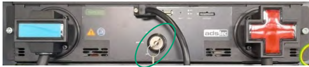
Abbildung 23: SRC4 Schlüsselschalter in Position „off“
